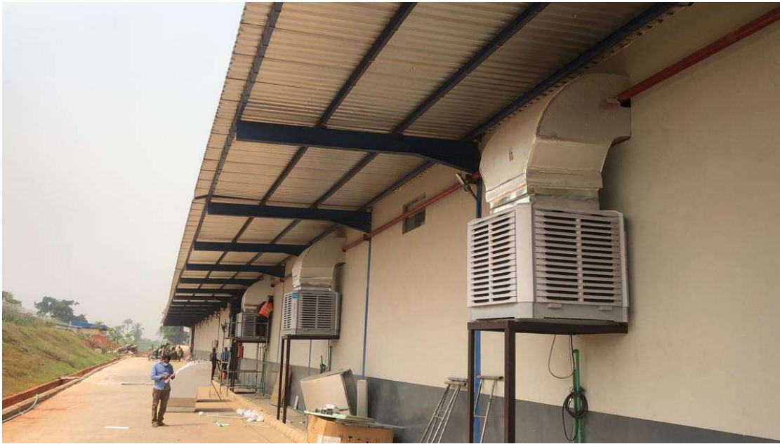
EVAPORATIVE AIR COOLERS (256,000 CMH)
