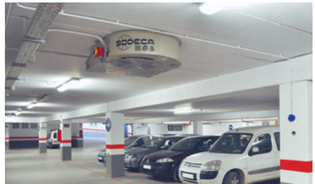
CI installed in car park
